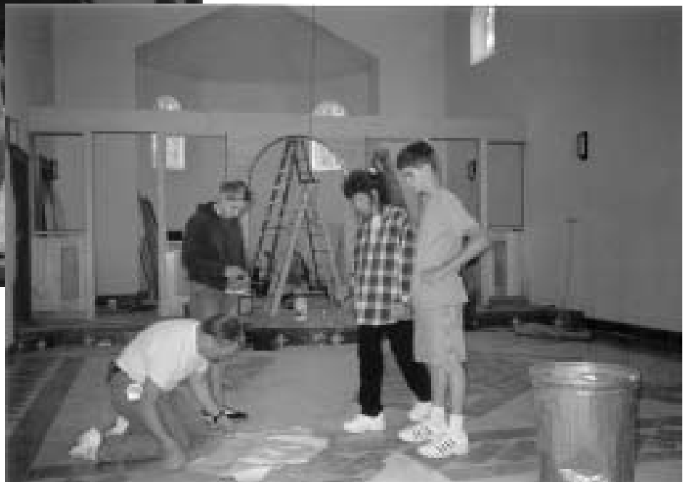
Members of the Schoonard family ponder a lay out of detail as they erect the Ico-nostasis .
