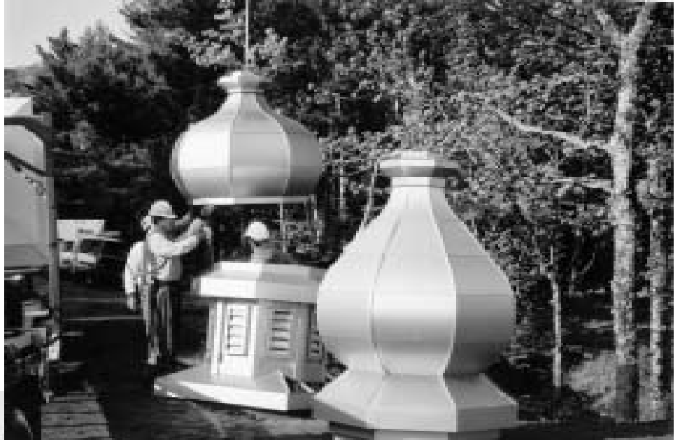
Workmen assemble the Dome for the Chapel of the Holy Cross of Sorrow and Suffering.
