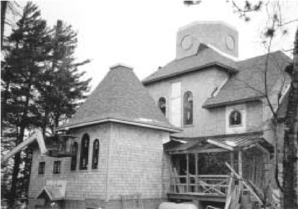
Workmen apply soffiting and facia to the nearly completed exterior of the Chapel of the Holy Cross of Sorrow and Suffering.
