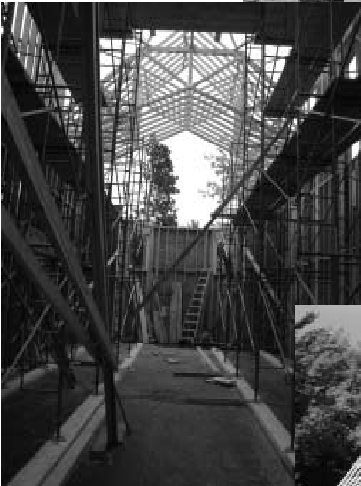
Interior of the Nave: Scaffolding provides safe footing for workers erecting Tower trusses, and for later insulation and drywall installation.
