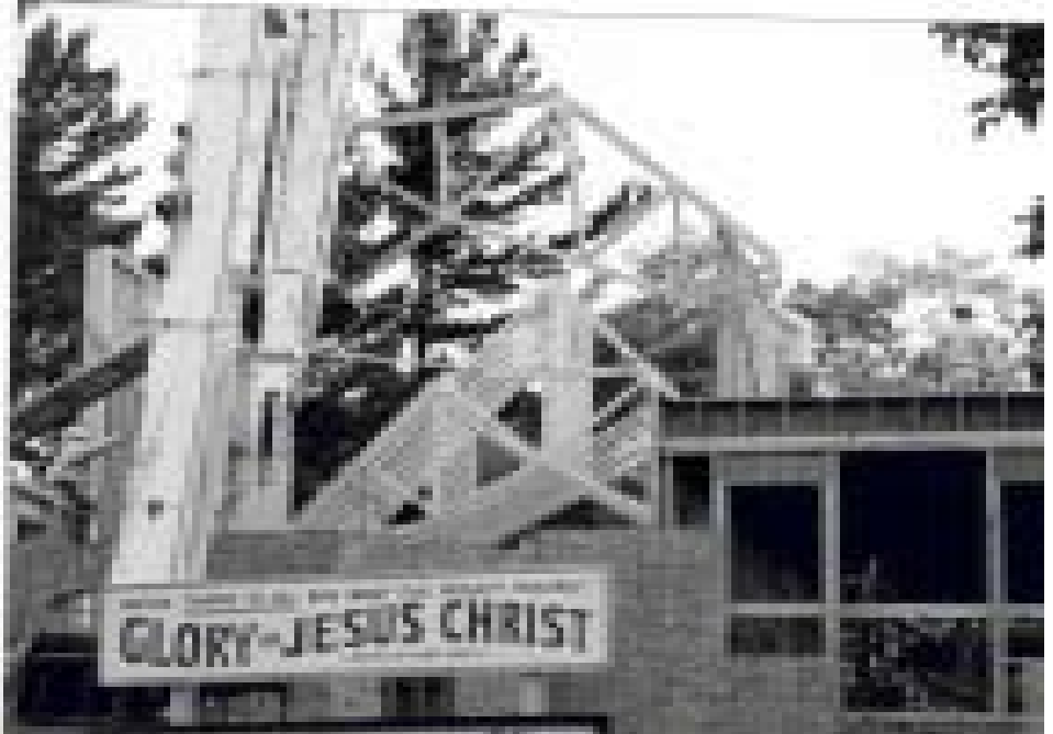
The Church roof begins to take shape as additional trusses are raised into place.
