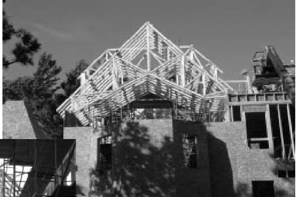
From the highway: Trusses for the Church roof and Tower in place.
