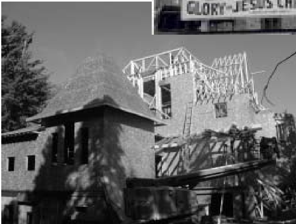
Beyond the sheathed roof of the Chapel of the Holy Cross of Sorrow and Suffering, the tower begins to take shape
