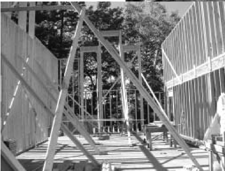
A sense of scale: The view from the Apse to the West windows of the future Church.
