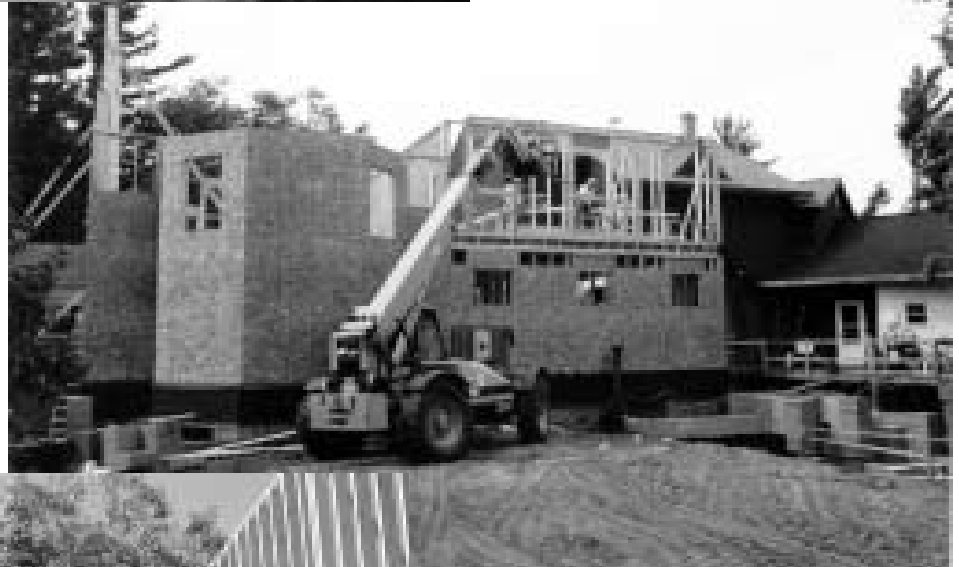
To the right of the Apse windows, framing for the Library Mezzanine partially obstructs the existing construction.
