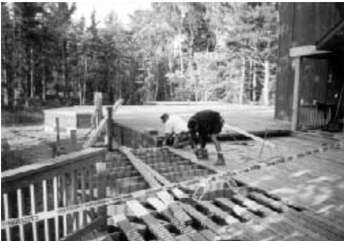
Day one: Dismantling the deck adjacent to our kitchen to accommodate bell tower excavations at the Northeast corner of the project.
