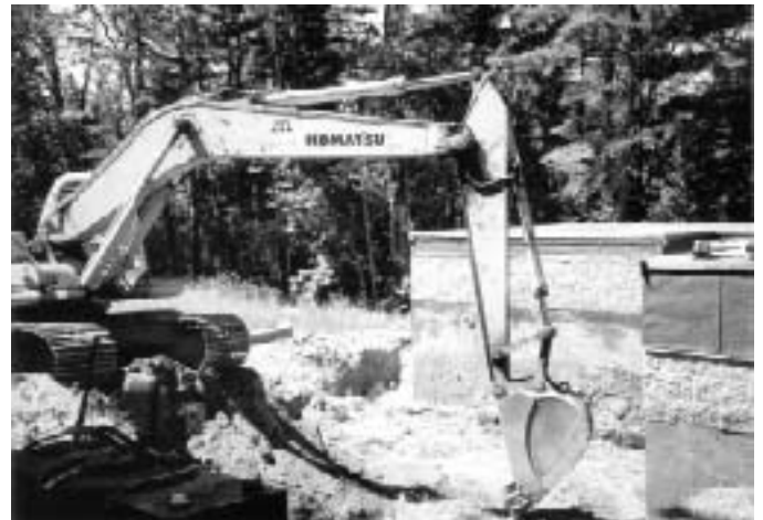
Southeast Corner: Excavating for the Chapel of the Holy Cross of Sorrow and Suffering.
